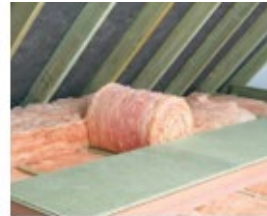
300mm+ Attic insulation
